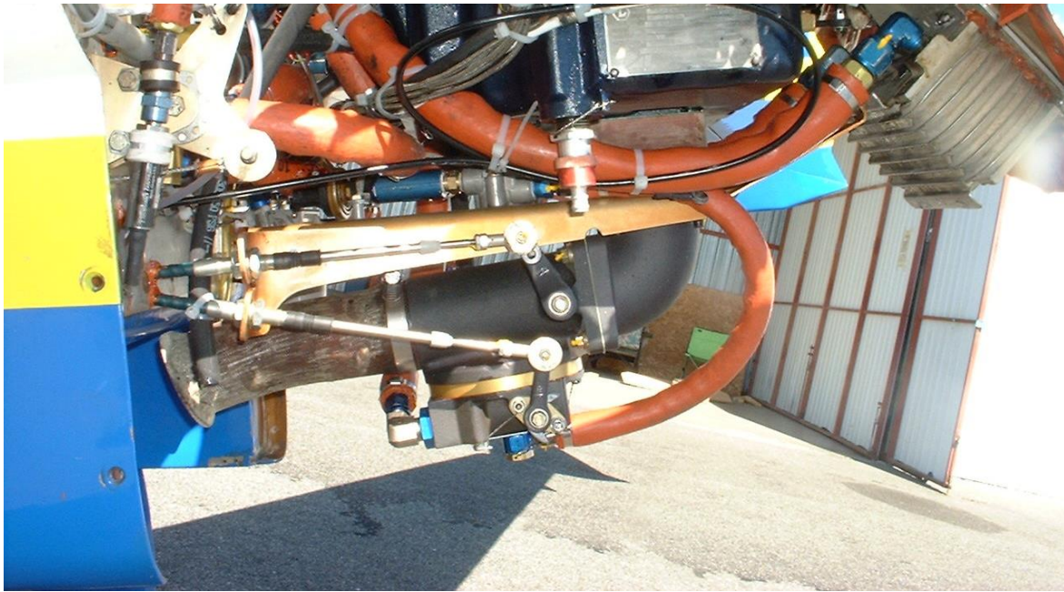
A Long EZ installation using an 85-degree elbow and phenolic spacers locates the fuel control into air inlet.
